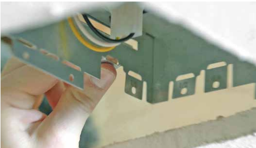
Holding tabs hold the fan from above the sheetrock
